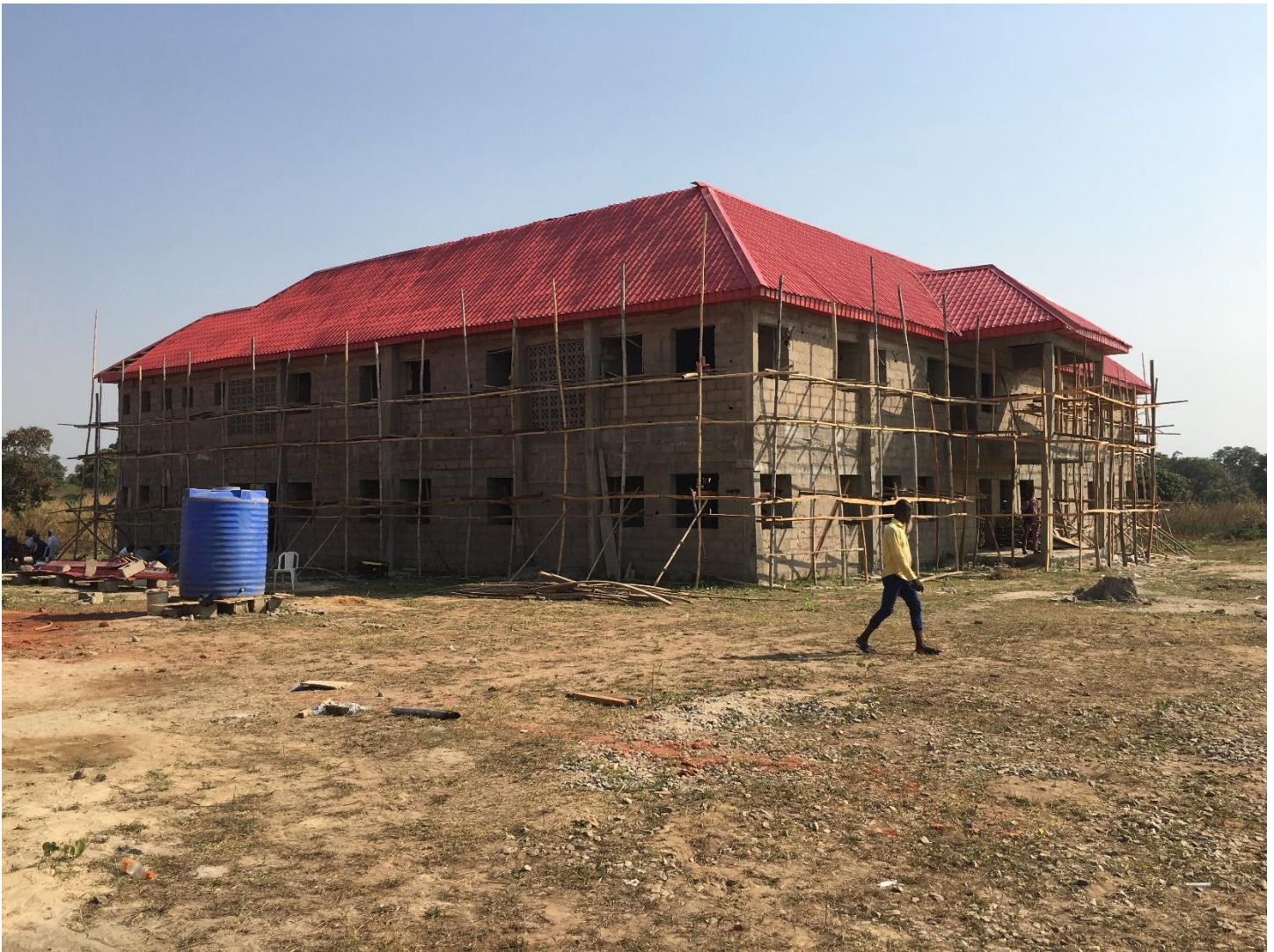
This view shows how large the Girls Hostel is. The roof looks beautiful and is about 95% completed.
